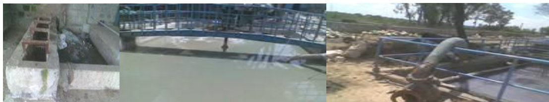
Figure 5. From left, screening bar, oxidation ponds with agitator and exhausting pipe (photographed by Oruko)
